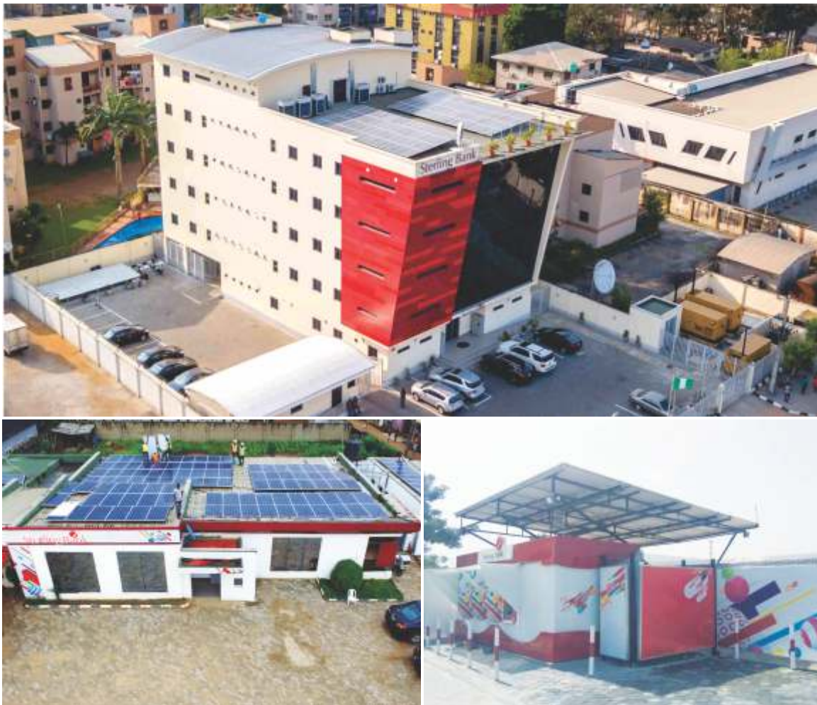
Top: The 45Kwh Hybrid Solar project installed at the Head Office Annex, Ilupeju, Lagos Bottom left: Deployment of hybrid power/ renewable energy at Magboro Branch, Ogun state Bottom right: Hybrid powered Offsite ATMs at Admiralty Way, Lekki, Lagos
